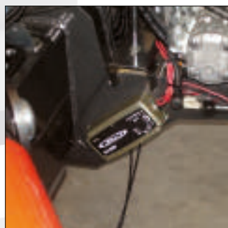
Maintenance battery charger, for endothermic engine ignition battery.
